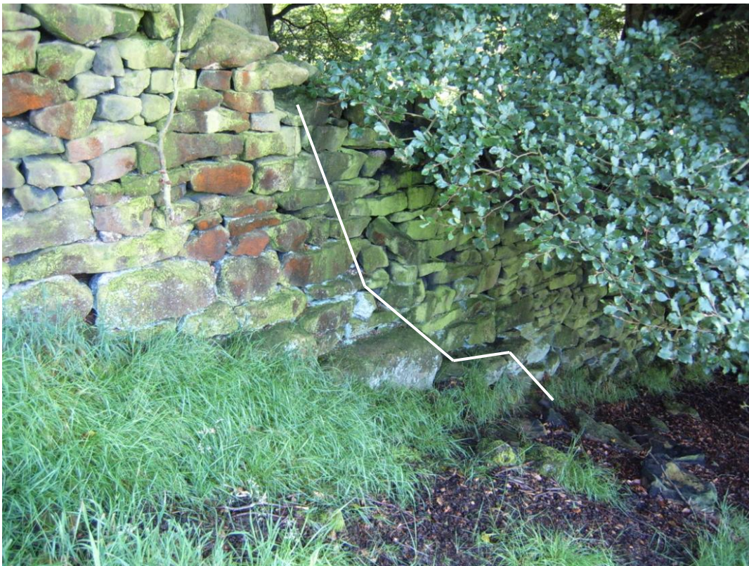
Fig 14: Photograph of the Northern (Bradley) enclosure boundary wall at the point where it meets the Eastern medieval wall. Notice the distinct change in construction pattern (white line), with a two or three possible orthostats used here although they are largely absent from the rest of this wall.
