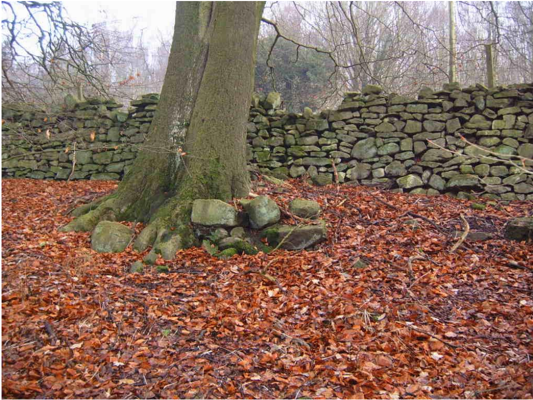
Fig 9: Part of the far Northern (Bradley) end of the Eastern wall, photographed from within the wood. Here orthostat rubble has been used to provide a solid platform for the later rebuild. The mature beech tree (250+ years old) growing through the rubble suggests that this section of the wall was rebuilt before 1750.
