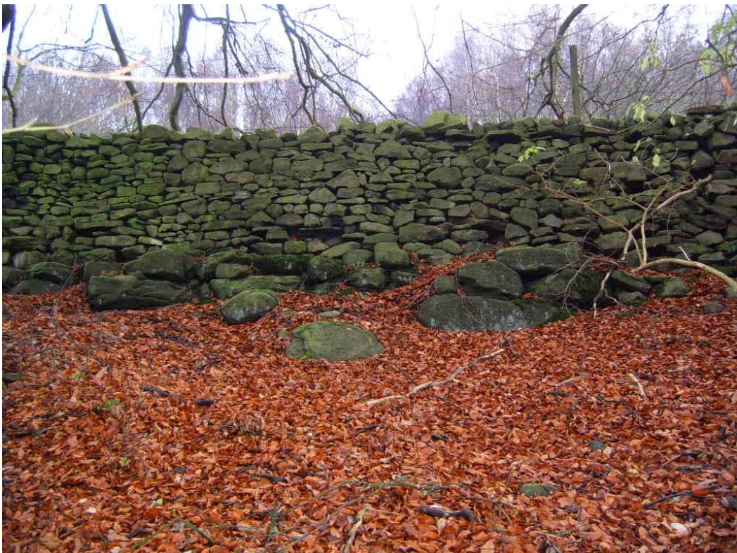
Fig 10: Part of the far Northern (Bradley) end of the Eastern wall, photographed from within the wood. Orthostats from the original medieval wall have been used as buttressing for the later rebuild.
