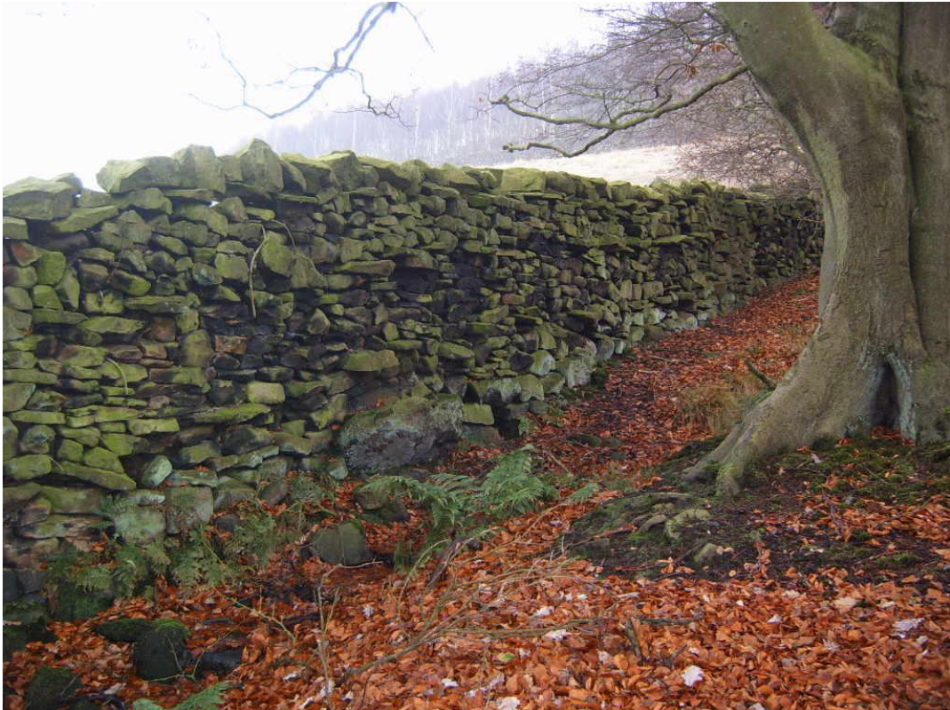
Fig 13: Another section of the Northern (Bradley) boundary wall, photographed from within the wood. Here the wall, descending a steep slope has two sets of throughs.
